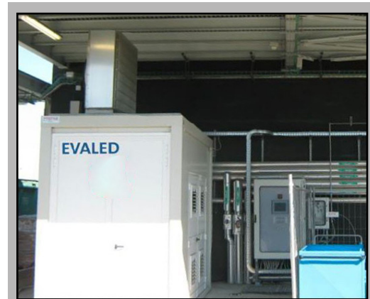
EVALED Vacuum Evaporator (Model PC F4 FF) installed at the laboratory has a small footprint of only 34 sq/ft.
