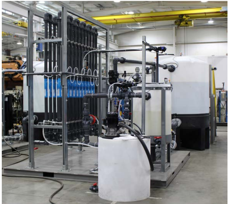
Pictured Above: PRAB Tubular Ultrafiltration system used to treat oily wastewater consisting mostly of used die lube and mop bucket/floor scrubber water. This system was custom designed with twenty-two Porex Tubular Membranes (1" in diameter by 6' long) that were vertically mounted to minimize floor space.
