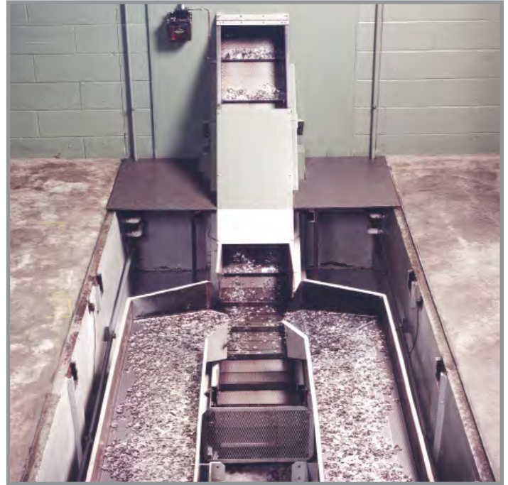
Twin in-floor oscillators with side discharge chutes merge sticky slugs and trim onto a Rigidized Pivot Belt™ to elevate and dynamically discharge scrap.
