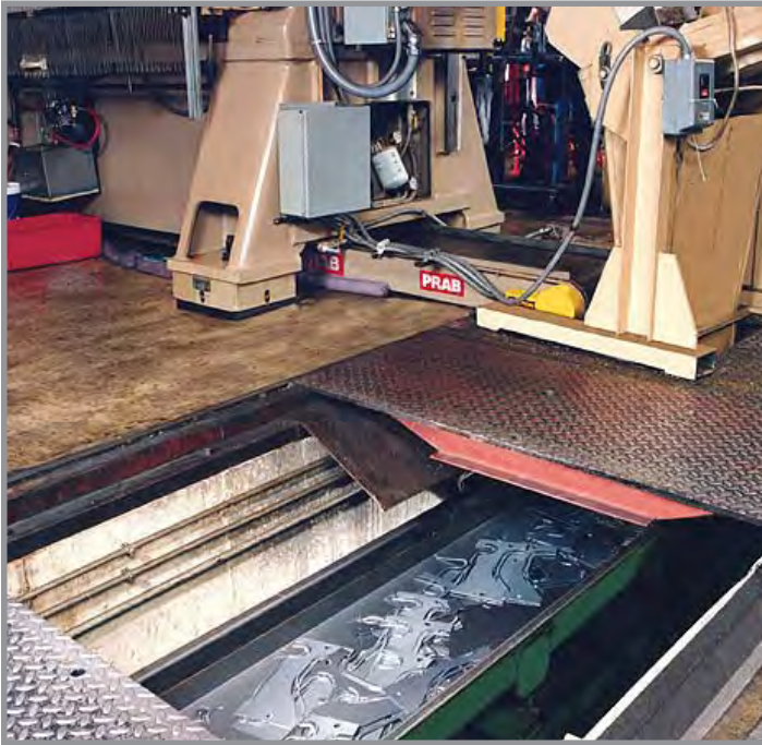
An under-press magnetic conveyor contains and transfers scrap, without spillage, down to an in-floor oscillating conveyor which also handles skeletal trim from a coil-fed scrap chopper.
