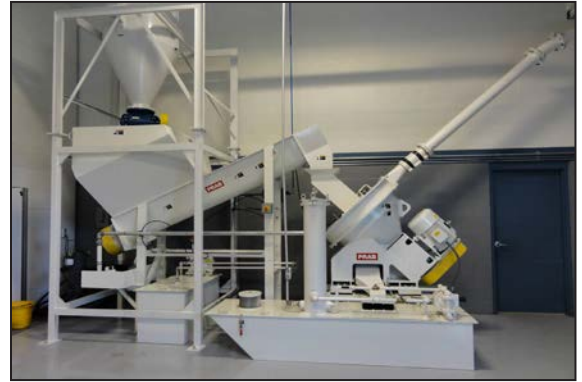
Pneumatic system feeds hopper to chip system and transports chips to outside silo
